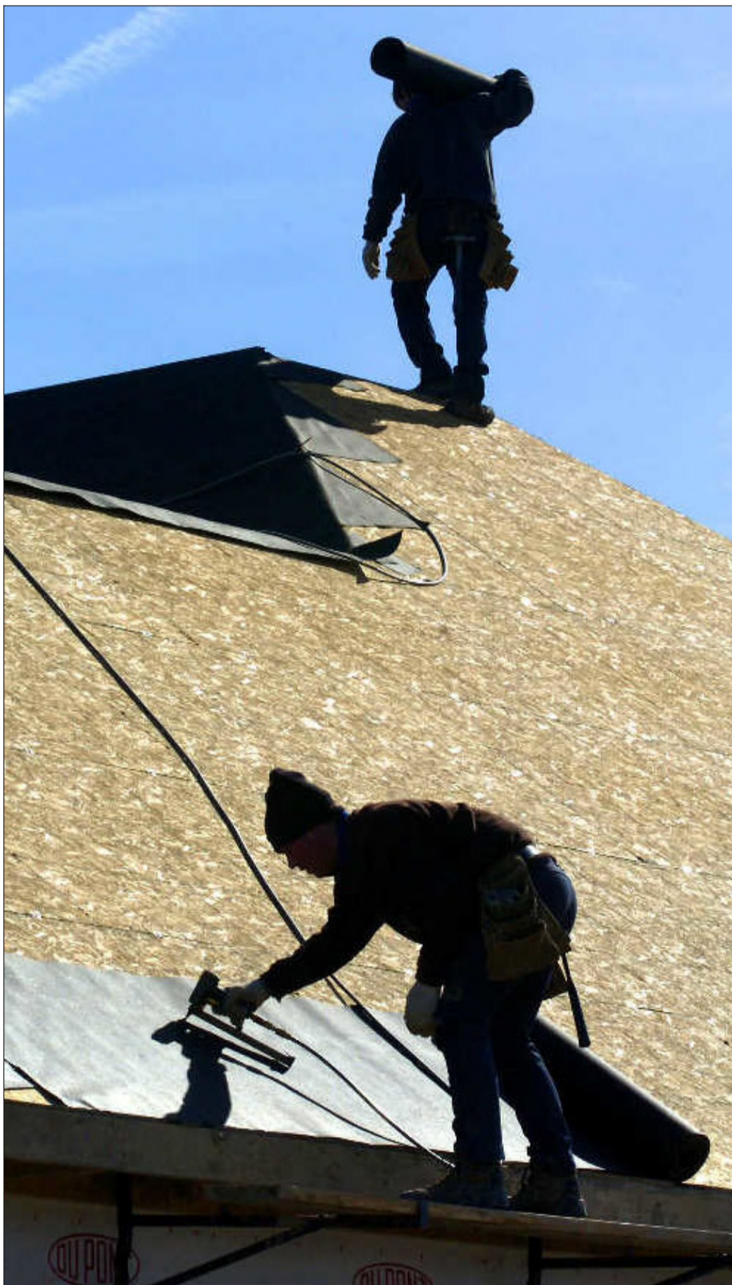
By Brian Tombaugh of The News-Sentinel An Amish framing crew from Lengacher Bros. works on the roof of a home this spring for Farmington Homes in Foxwood addition, off Wheelock Road.
